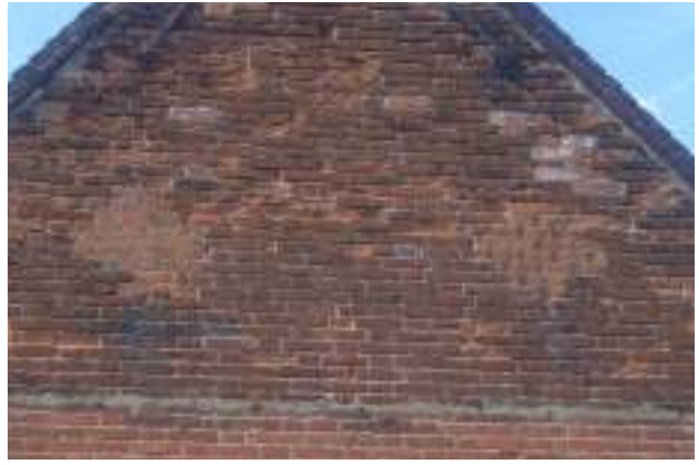
Blocked diamond pattern honeycomb ventilation openings on south gable – closed off by inserting additional bricks into the honeycomb openings using cement mortar, suggesting done circa 2000
