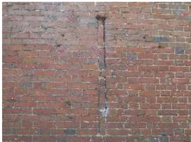
Blocked ventilation opening on east wall – crudely blocked from outside by stuffing space with upended bricks secured with minimal lime mortar, suggesting inter-war work
