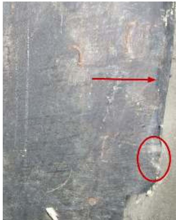
Another view of chamfered edge (arrowed) with run out stop (circled) at bottom
