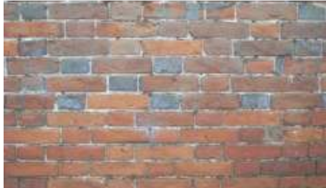
Flemish bonded brickwork to walls above plinth – alternating stretchers and headers in every course.
