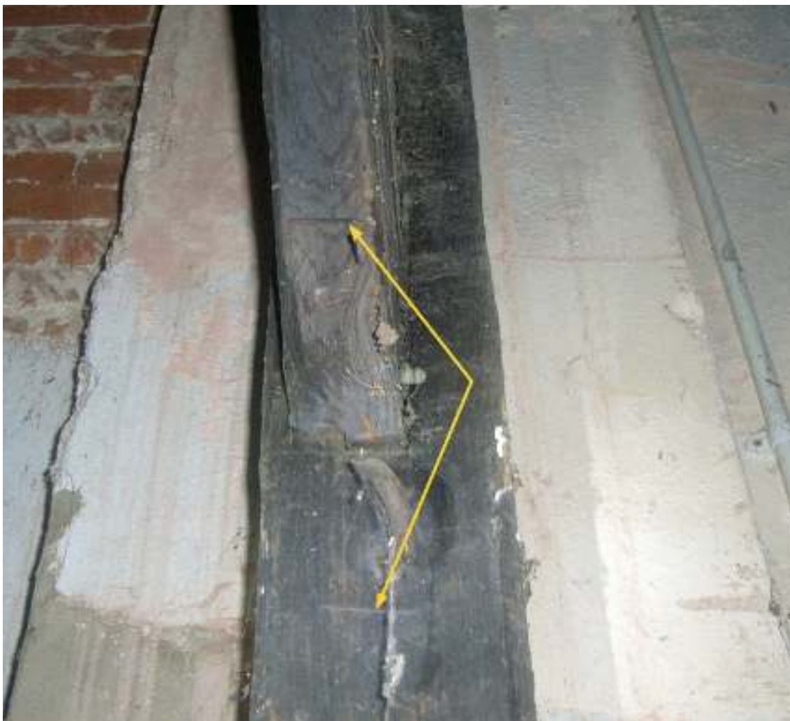
Carpenters marks (arrowed) – in this case for joint number 1. The two stopped chamfers can also be clearly seen on both edges of the post below the joint and can also just be seen on the bottom of the brace – although not visible in this photo, a separate pair of stopped chamfers start on the post just above this joint, and the tie beam itself has matching chamfers albeit larger.
