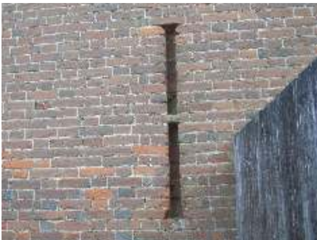
Blocked ventilation opening on north wall – carefully blocked from inside using bricks laid on their sides and bedded in lime mortar, suggesting late 19 th century work
