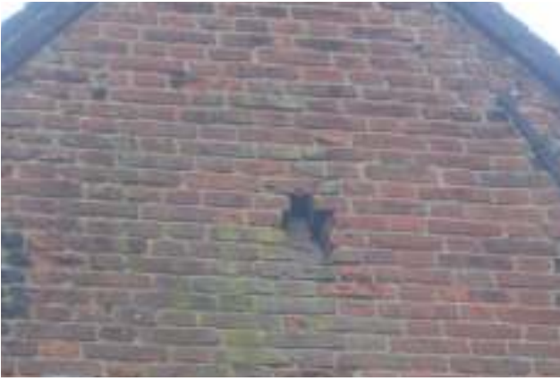
Blocked ventilation opening on north gable – crudely achieved by covering the opening internally with modern building materials, suggesting circa 1970s work
