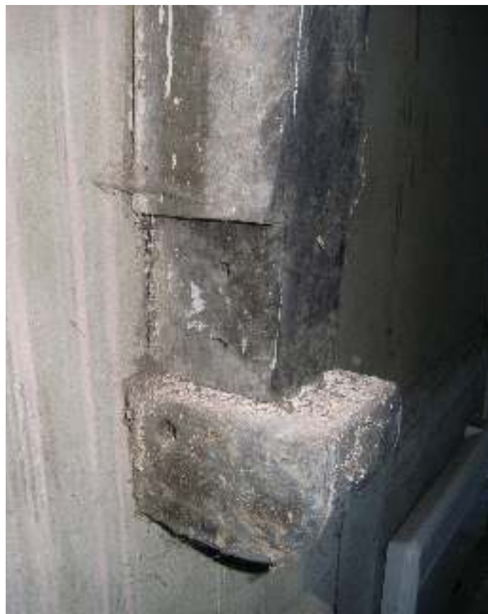
Foot of a braced tie beam showing that the vertical post was originally part of a different building
