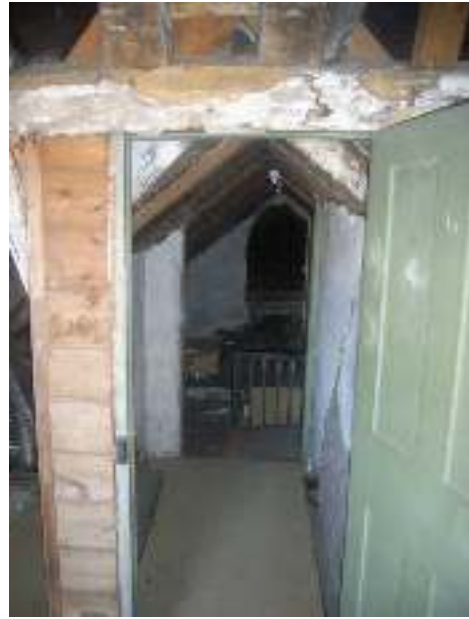
View back through 'tunnel' to the landing with the opening into the roof space of a rear wing beyond.
