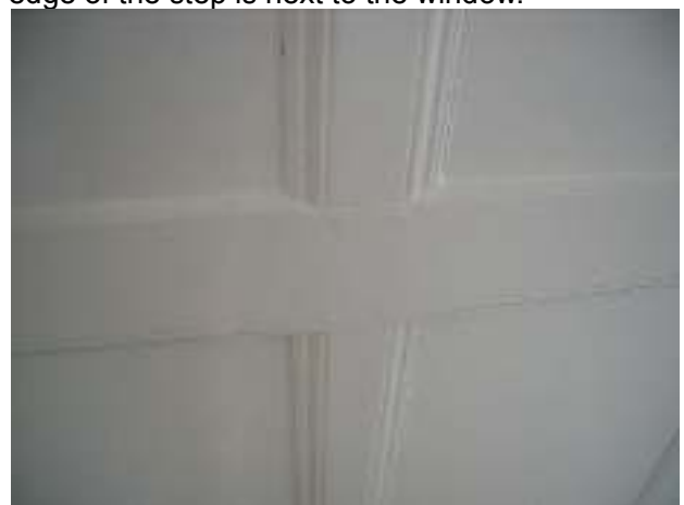
Close-up of door in left of previous picture – this was originally part of a full height panelled wall. The panelling is hand-made and could pre-date the building as currently comprised.
