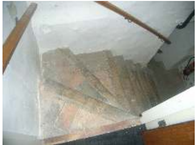
The cellar stairs were almost certainly constructed at the same time as the staircase they run under – both are consistent with circa 1800 work.
