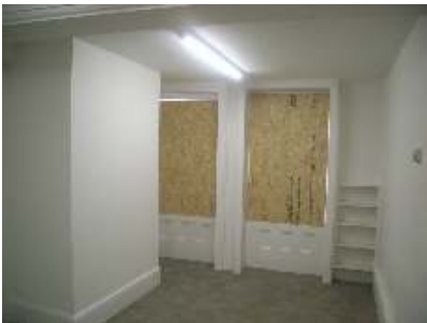
Inserted chimney backing onto the hallway that already reduces the width of the room by 6ft. This chimney matches that in the large back room within the middle rear wing. The very deep alcoves allied to a moderate breast width are typical of circa 1800 work, but in this case leave one window almost completely obscured!
