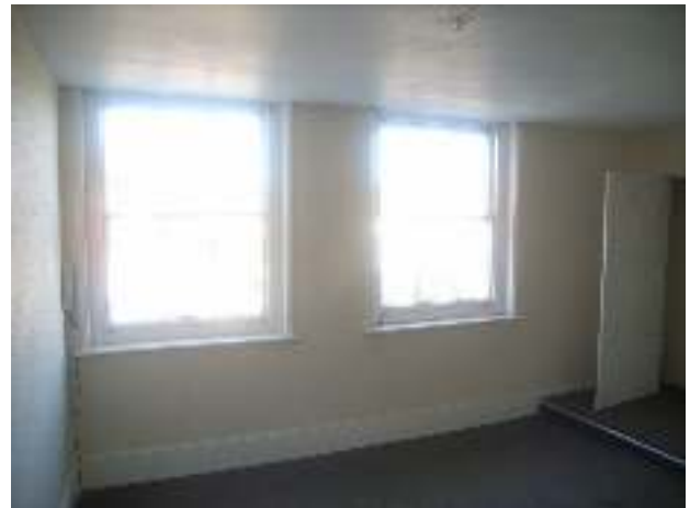
The original party wall, between what is nominally numbers 12 and 13, was removed to extend the middle front room over the hallway (created out of the southernmost ground floor room). In the above picture, the party wall used to be where the edge of the step is next to the window.
