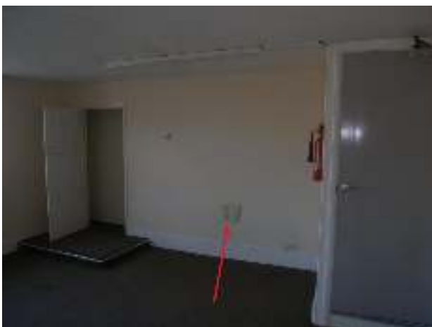
Removing the old party wall gave the middle front room access to the chimney running up beside the ground floor hall, enabling a fireplace to be provided (now removed – location arrowed).
