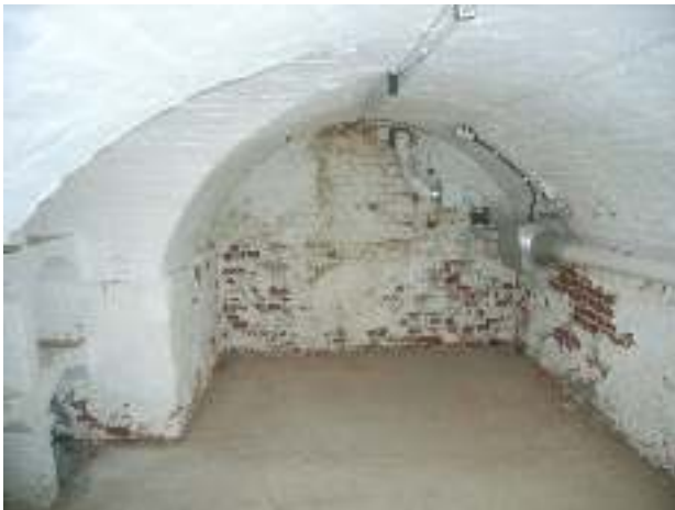
Second cellar – typical domestic scale cellar dating from the late 18 th /early 19 th century.
