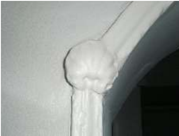
The mouldings on the arch at the end of the hallway are heavily obscured by thick paint but include shell motifs and are consistent with work from circa 1800.
