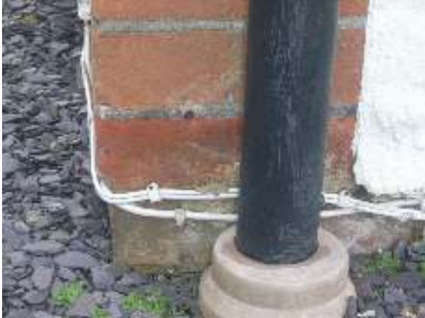
Brickwork on front corner overhanging the brickwork used to form the base of the walls.
